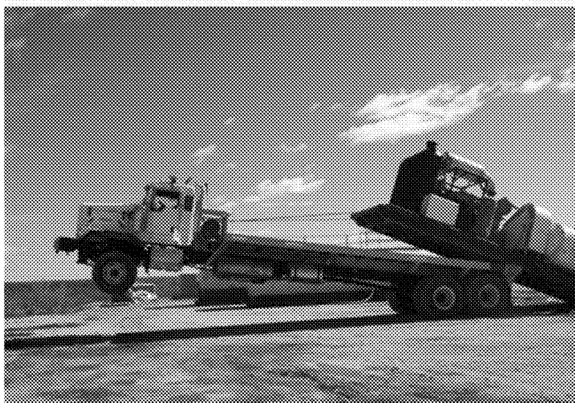
FIGURE 8- Stress and force balance in the tension of the cable of the winch truck and the load.
